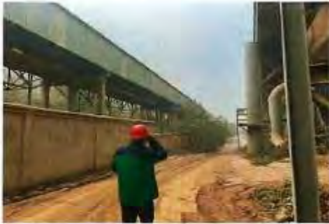
ADA002 中细破车间出料废气排放口 B
