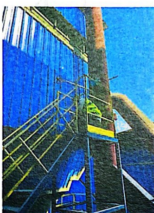
1#包装机排气筒
